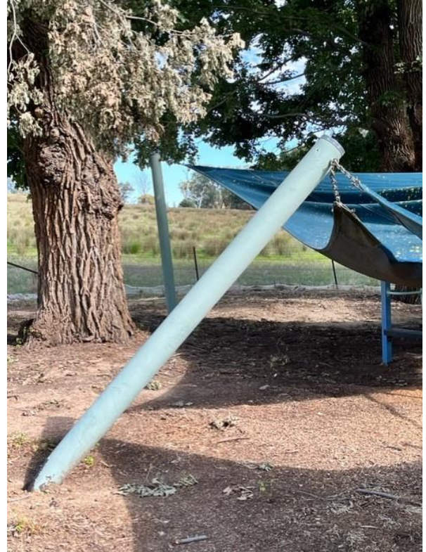
Storm damage to Shade Sail
